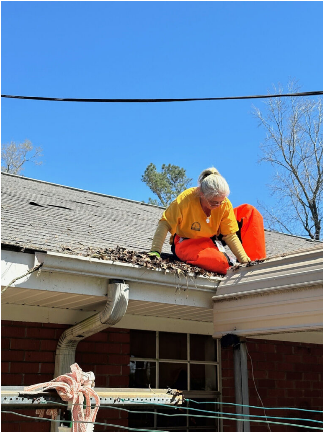
Sandy Henderson, a volunteer from Pearl River Association, cleans debris off a roof of a home damaged in the March 15 tornadoes near Tylertown. (Photo credit: Tony Martin)
